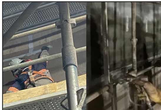
Stripe coating weld seams and spraying first coat of ARC S5 Coating.
